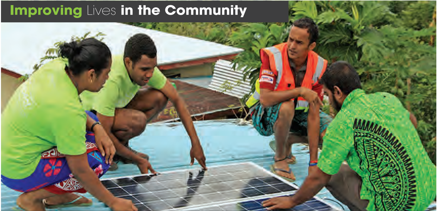
In Fiji, BSP delivered 6 projects to schools, installing Solar Lights and contributing to improving lives in the community. Pictured, BSP Fiji staff working with contractors to install a solar panel at Nailuva District School.
